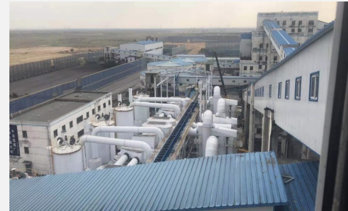
-30mm Coal Separation (9.0 Mtpa, Shangkaimiao Coal Mine)
