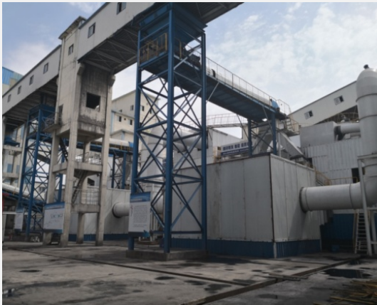
80-0mm Mixed Coal Separation (6.0 Mtpa, Yushujin Coal Mine)
