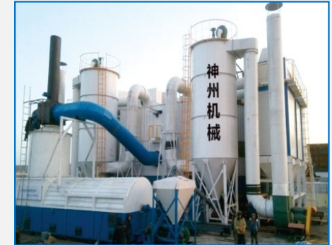
Drying-Dry Separation System
